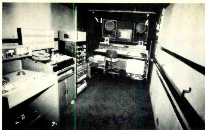
Interior of Rocshire's API/3M-equipped remote recording truck.
