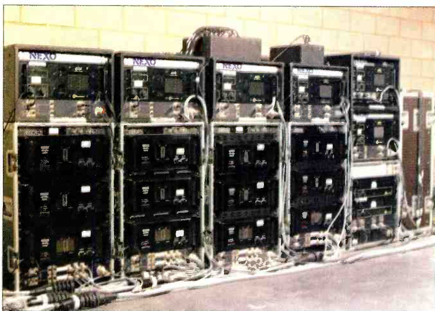
All of the signal sources were routed first to the main racks and then distributed from there to the others via multicores.
