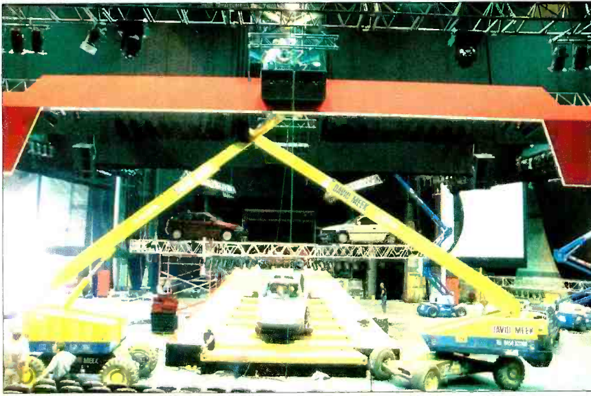
The speakers were flown at 22 motor hoist positions around the hall's 43 feet high ceiling, which comprises a network of steel grids with access for the riggers.
