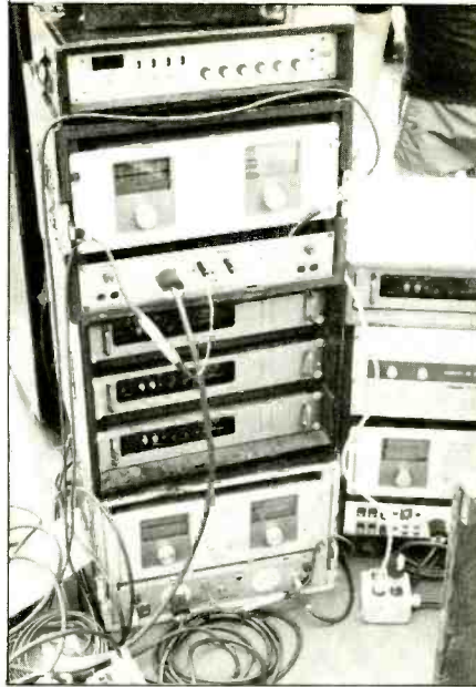
Figure 6: Modular's power amplifier racks house Carver PM1.5s for mid and high amplification. Phase Linear D-500s power the LF components.
