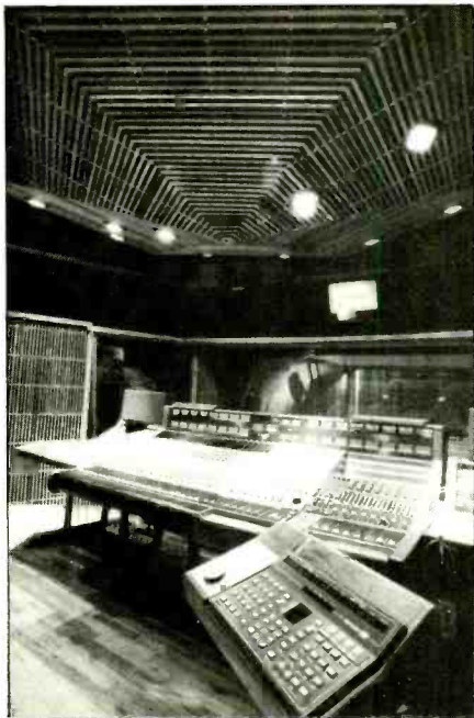
An unusual feature of the control room acoustics is the pyramid-shaped ceiling, designed to reduce standing waves.
