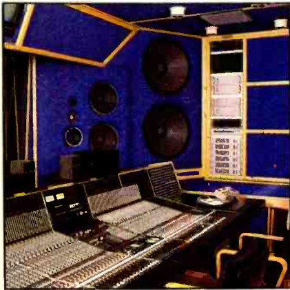
Closeup of Control Room A's right-hand monitor bank.
