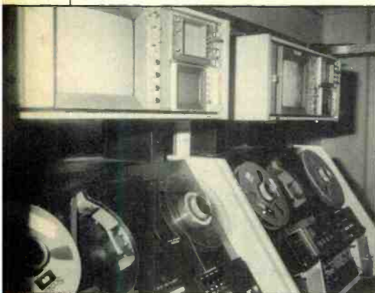
Within the facility's video control room, two interlocked Ampex VTRs provide picture playback, and the PCM audio.
