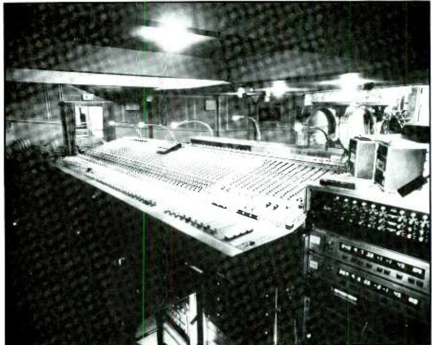
An Autograph installation at the Shaftesbury Theater in London showing the Cadac console and the outboard signal processing rack.
