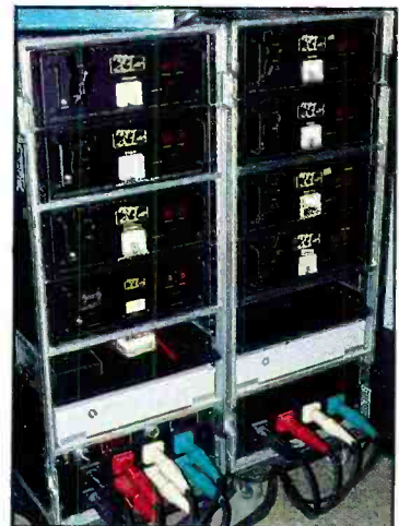
Figure 11. A power distribution panel for the stage ac, including Juice Goose line conditioner/voltage regulator devices for each circuit.
