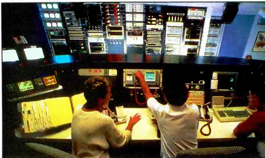
Photo 1. A digital audio control room used to route digitized audio to the transponders coordinating the uplink and downlink.
