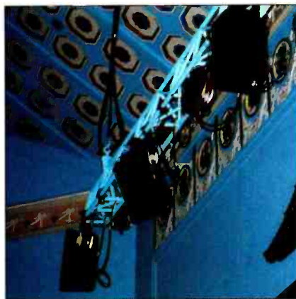
Figure 1. The center bridge truss, hung from the ceiling in front of the stage, holds three Meyer UPAs and three Tannoy 3859-R coaxial speaker units.
