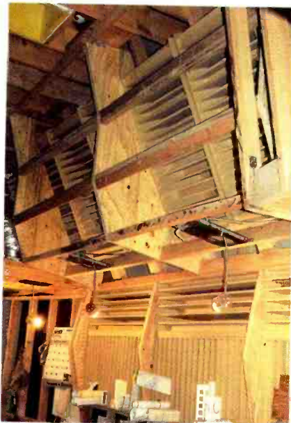
RPG Diffusers along the rear of control room wall.
