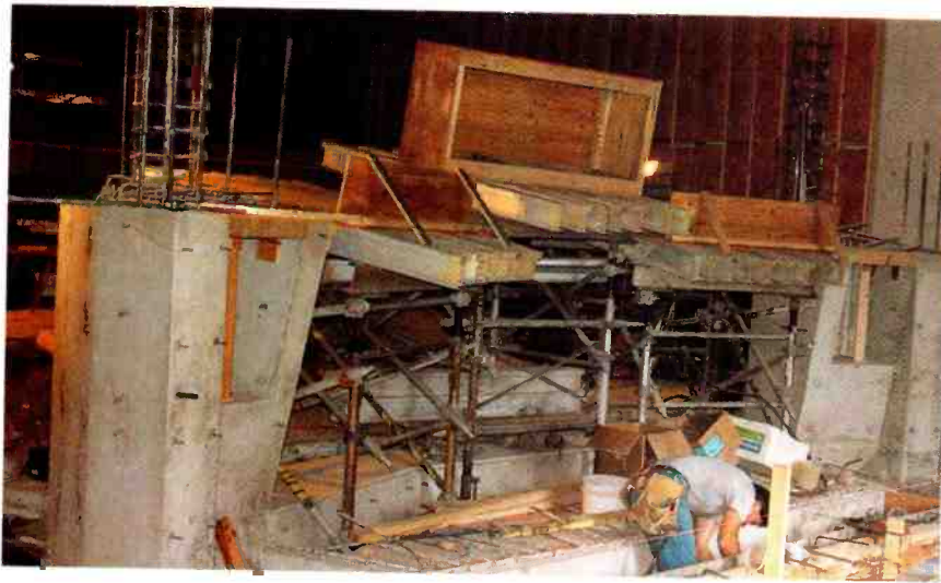
Poured concrete control room front monitor wall, with console wiring trough and PVC conduit.
