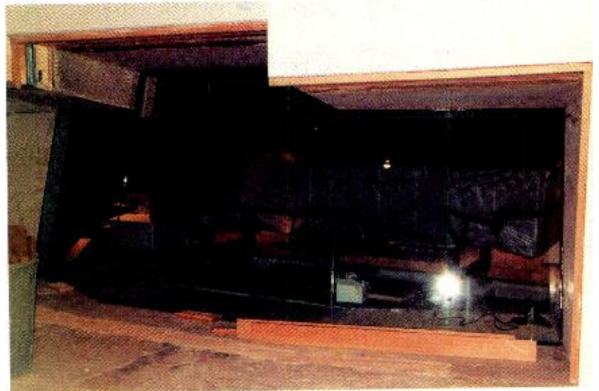
View of Studio X control room glass from the studio room. Note that the glass goes all the way to the floor. SSL is in place.
