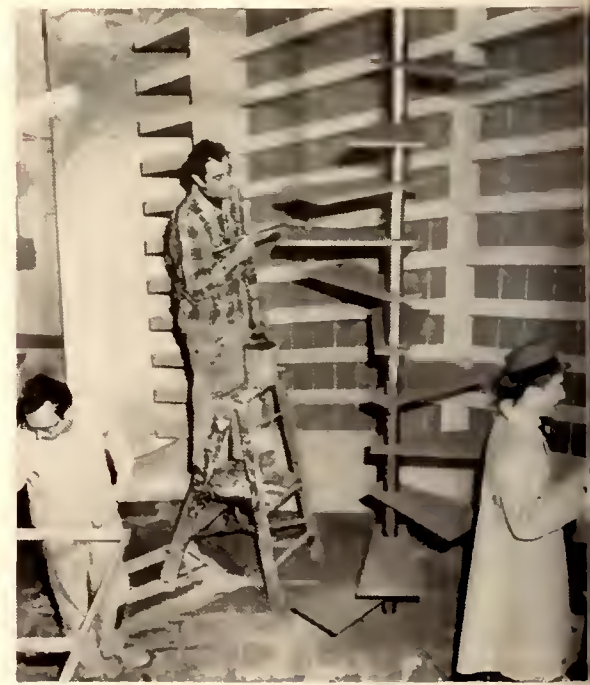
Scenery construction, supervised by Wes Doyle, cost $5,000 in addition to usual $1,400 for normal set design. Rotondo was commissioned to design sets for the "house"
