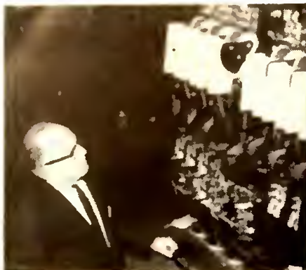
Robert J. Sinnett, Director of Engineering for WHBF Radio and TV, checks emergency power supply automatic switching panel at WHBF-TV transmitter.
