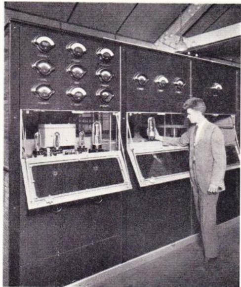
The first three panels of the transmitter
