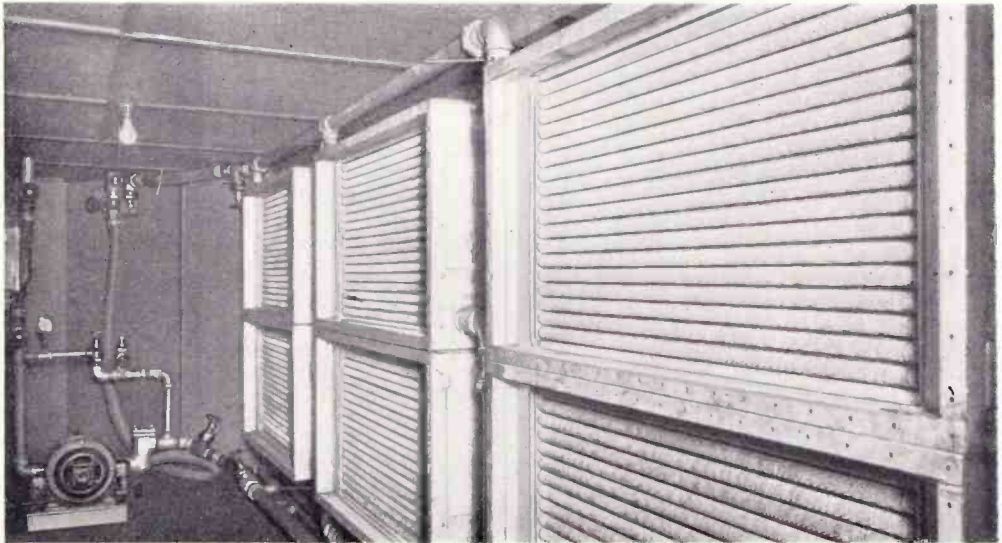
Cooling water from the tube jackets in turn gives up its heat to the air blown through these radiators
