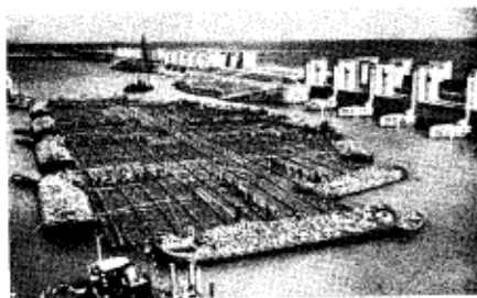
A "mattress" being weighted with rocks to sink it, to protect the bottom from erosion.
