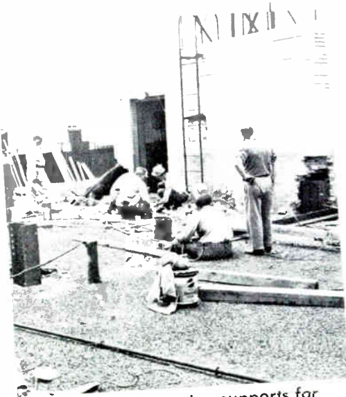
Workmen preparing supports for TV tower on top of the First National Tower building.
