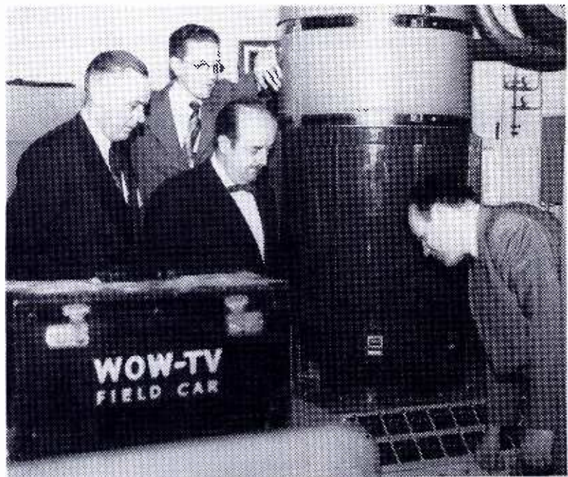
WOW-TV management personnel watch RCA Field Engineer Frank Porter as he makes last minute adjustments in transmitter room before WOW-TV increased to 100,000 watts "Maximum Power," Tuesday, February 24. Pictured are left to right General Manager Frank P. Fogarty, Chief Engineer Bill Kotera and Assistant General Manager Lyle DeMoss. (Details on page 1 of Television Section.)
