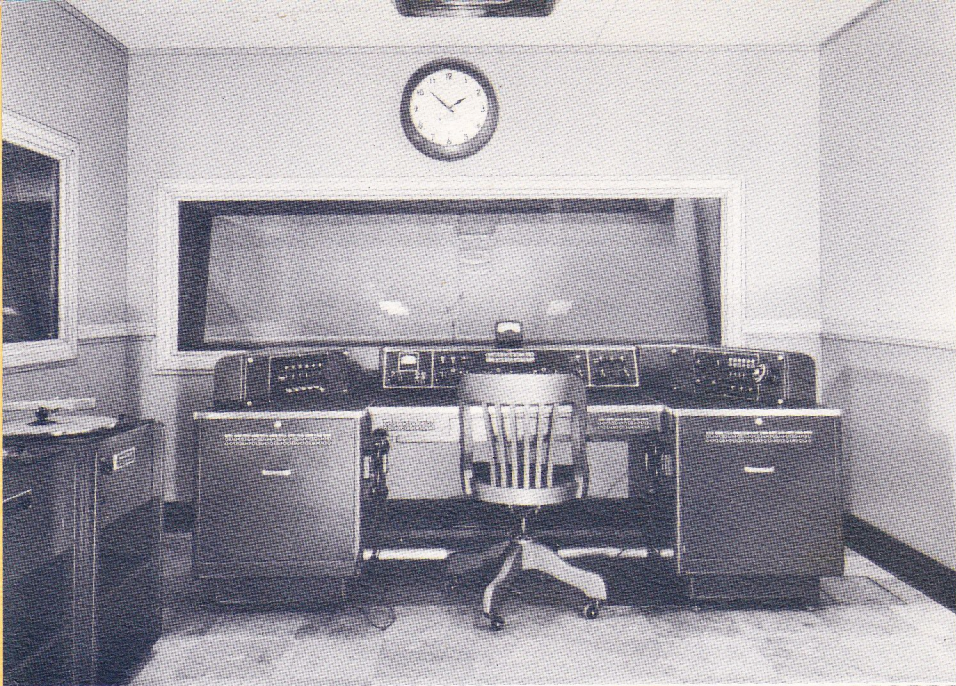
All WTMJ programs clear through this sub-master control room. Station W55M has similar equipment in Radio City.
