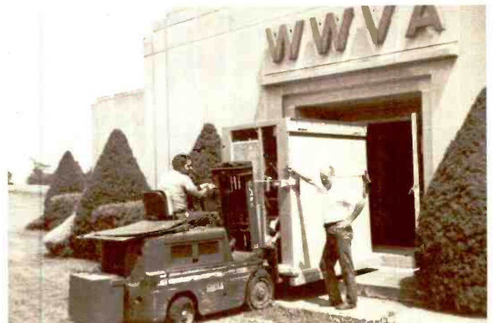
In July 1969, when the new 50,000 watt transmitter was installed at the WWVA St. Clairsville transmitter site, it took men and machines to handle the big job.
