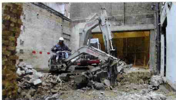
5. The heavy plant moves in. It was a four-month job running from February to June. The heavy rain during February caused some flooding because the water table is high here. Additional drainage was added as part of the rebuild. Also, consideration had to be given to one of adjoining walls as it belongs to a neighbour—before starting we invited the locals in to look around and to explain what we were going to do. (Week 5)
