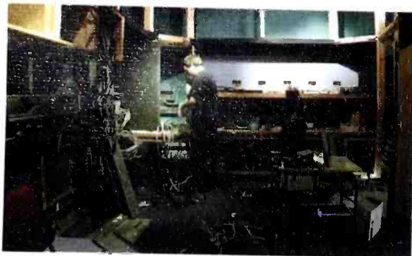
2. The machine room being dismantled, which was originally built c1984 in the space which was the side entrance to the building. (Week 1)
