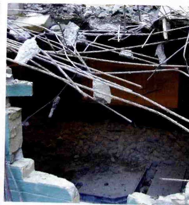
4. Looking into the stripped control room from the outside world prior to demolishing the walls and ripping up the foundations. (Week 4)
