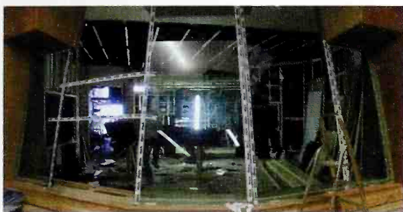
8. The front of the new control room with its bigger window. The window sits beneath a structural girder that limits its height. The challenge here was to work around this to improve the lines of sight between control room and studio. (Week 15)
