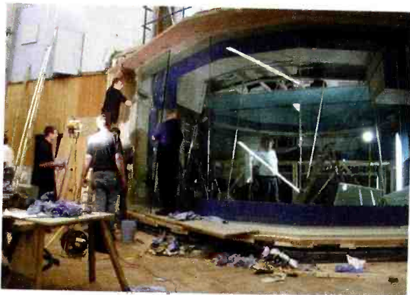
11. The second layer of glass going into the control room window. (Week 18)
