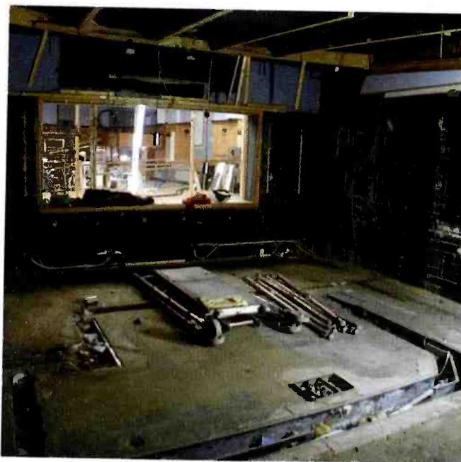
3. Emptied of equipment, you can see the control room cable trench and the studio, which became a temporary workshop and store room during the project. (Week 2)
