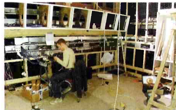
10. Equipment being reinstalled in the equipment room. It is more than twice the size it was before allowing for future expansion so there are a lot of blank panels. There are so many formats coming and going right now that we need a big space where people can bring stuff in. (Week 16)
