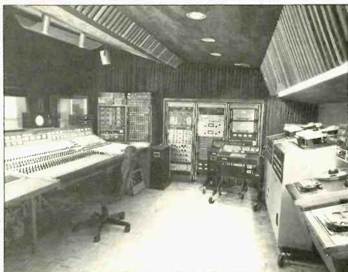
Control Room B
