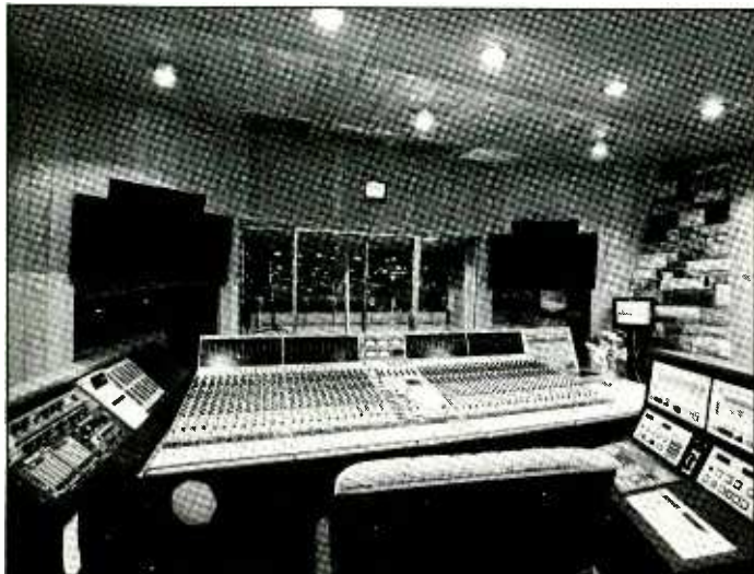
Eastlake control room
