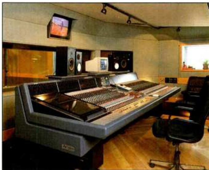
Control room at Westside
