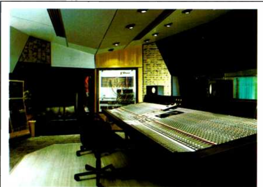
Control room studio 1 with SL9072-J console
