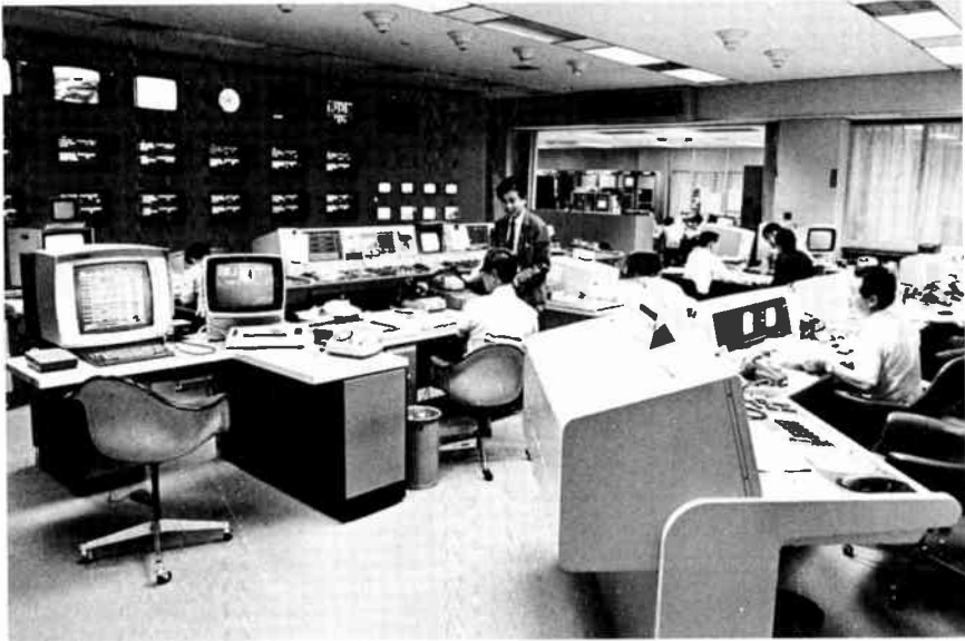
Figure 10-9 Transmission control room at the NHK Broadcasting Center. (NHK)
