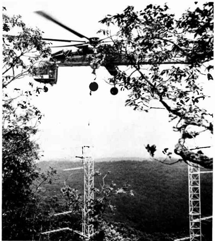
FIGURE 8-3 Installing cable head-end antennas can be a major task involving heavy equipment, expensive transport systems such as helicopters, and specially trained construction crews. (NCTA)
