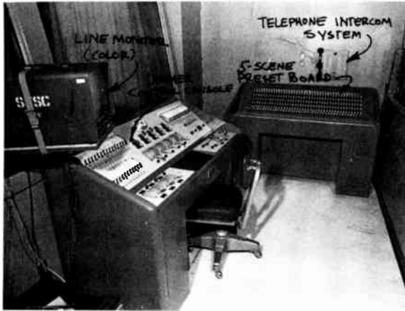
8-10 Lighting Control: The lighting control board consists of the dimmers and their preset controls, through which a variety of lights can be adjusted for their intensity either individually or in unison, depending on how they are patched.
