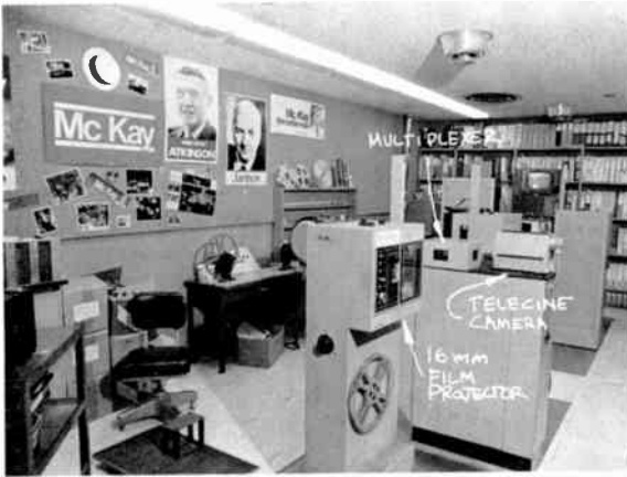
8-13 Telecine Room: Telecine contains the film islands, consisting of film projectors, slide projectors, multiplexers, and television film, or telecine, cameras
