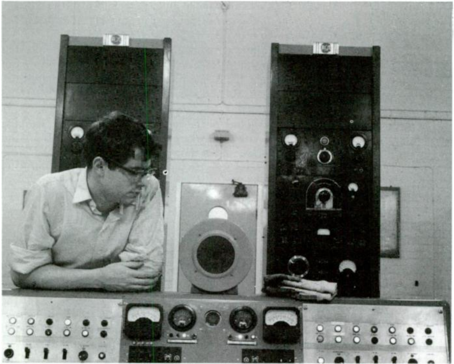
Figure 14.6 The original RCA transmitter control unit at Woofferton. Programme keys modulation meters in the centre of the desk with General Electric noise distortion and measuring equipment behind. Note the gloves for wave-changing on top of the desk
