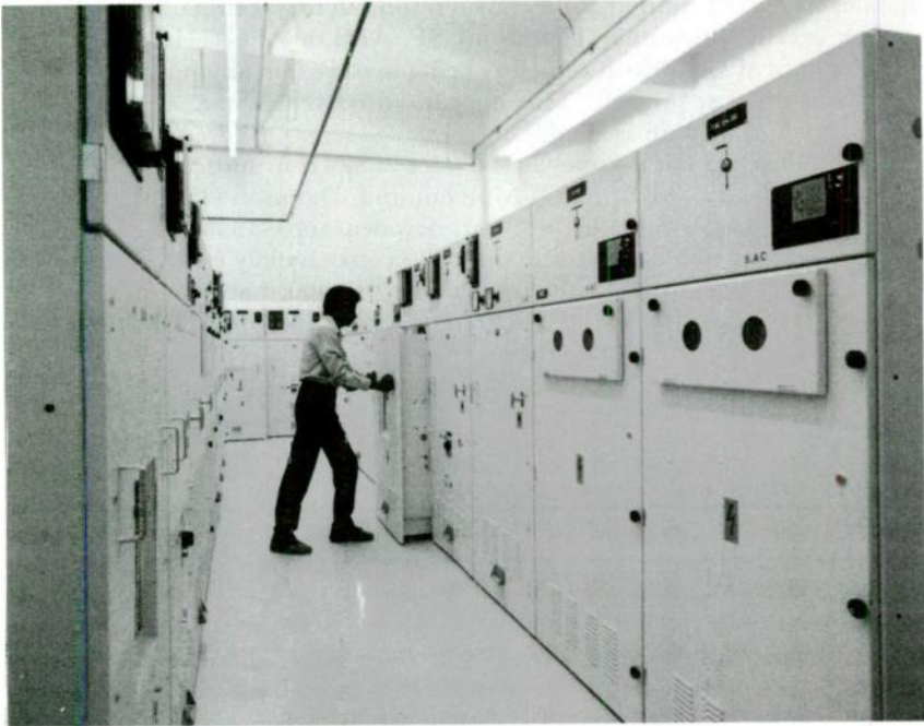
Figure 30.2 Transmitter station power control room at Qasr Kherane, Jordan
