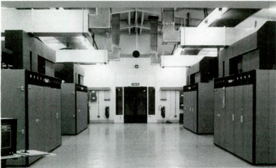
Figure 14.7 The Woofferton VOA relay station with four additional 300 kW B6124 short-wave transmitters added in 1987
