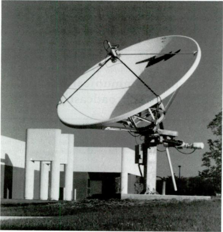
Figure 17.1 4.5 m C & Ku satellite dish in a downlink installation
