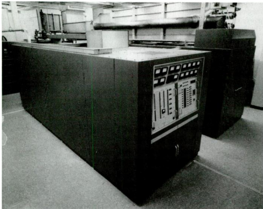
Figure 28.1 Continental 420B 500 kW shortwave transmitter installed at VOA, Greenville, USA
