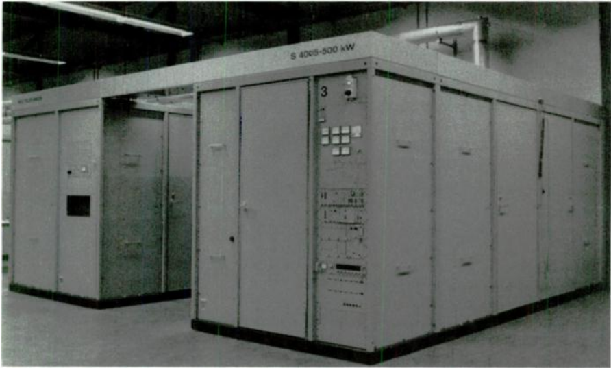
Figure 22.1 500 kW shortwave transmitter S4005 installed at Flevoland, the Netherlands
