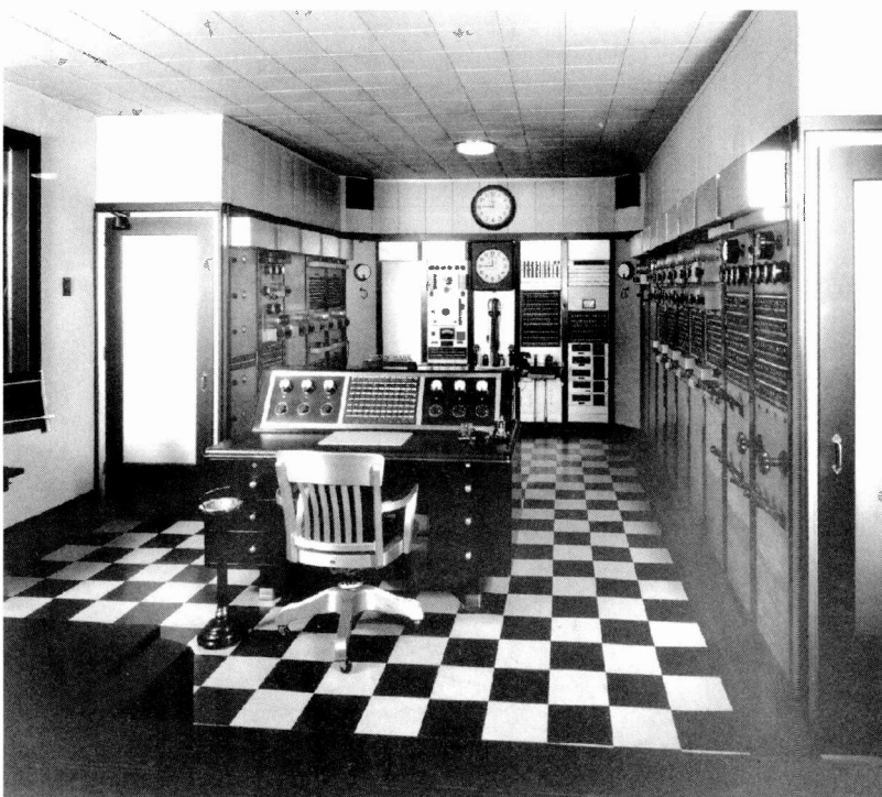
KDKA was proud of its heritage as a radio innovator and built state-of-the-art facilities, as reflected by this Master Control room.
