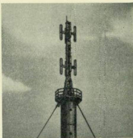
Close-up of the Sutton Coldfield transmitting aerial
