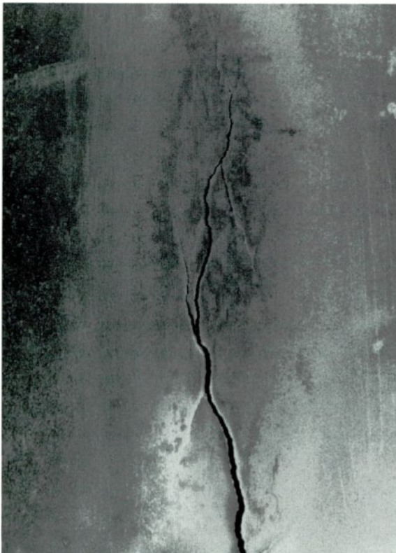
The crack is first sanded to clean the surface and prepare it for soldering.
