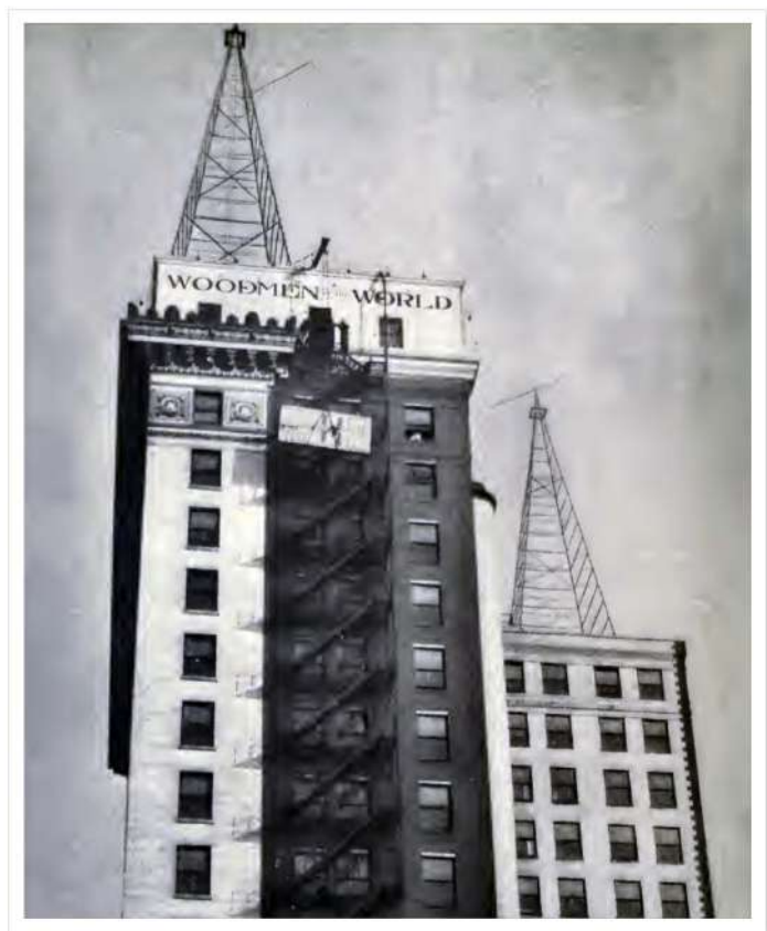
1923 photo of WOAW's new studios and towers atop the 18-story Woodmen of the World Building. The studio's huge pane of glass is shown here being hoisted upward for installation.
