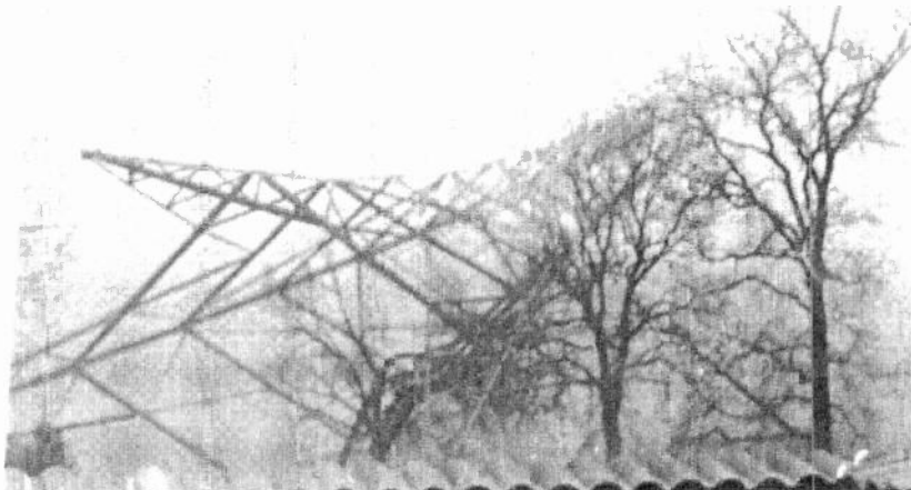
Demolition crews remove WGN antenna towers in preparation to move the transmitter site.
