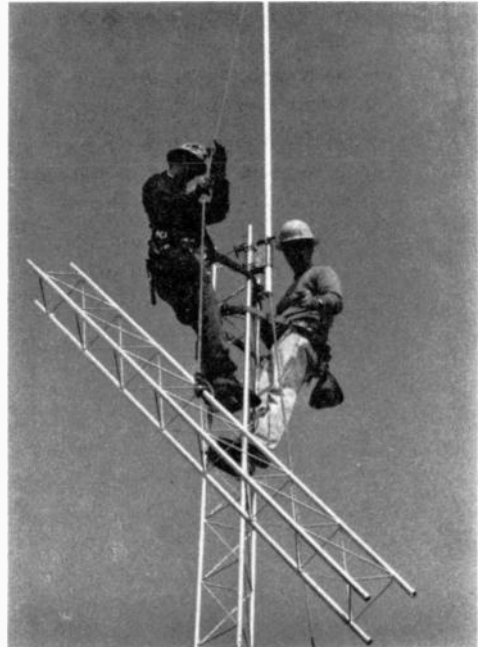
Fig. 14-9 — The assembly of tower sections is made simple when a gin pole is used to lift each one into position. Note that the safety belts of both climbers are fastened below the pole thereby preventing the strap from slipping over the top section. (Photo by K1THQ)
