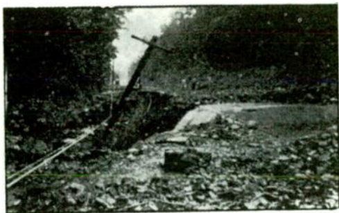
This is the type of flood washout that took communications with it at Ithaca, N. Y., in 1935.
