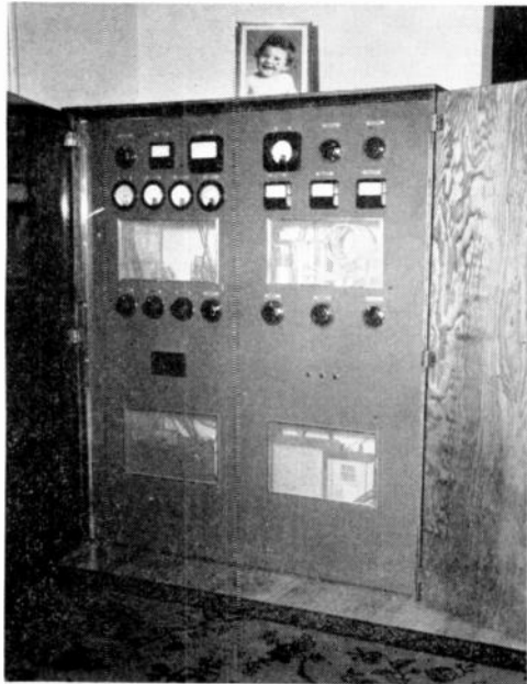
Fig. 11-12 — Opening the doors of the transmitter cabinet reveals this neat rig. Wire screen surrounds the transmitter and helps in the reduction of TVI.
