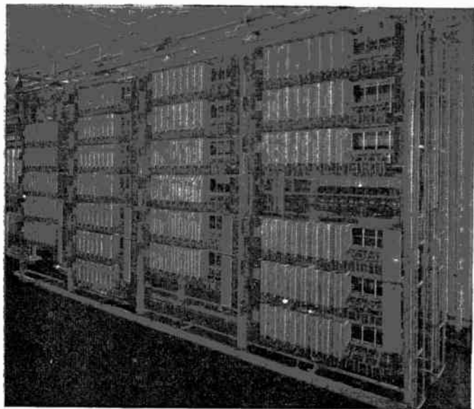
FIG. 7,668.—Step-by-step connectors mounted on switch frames.
