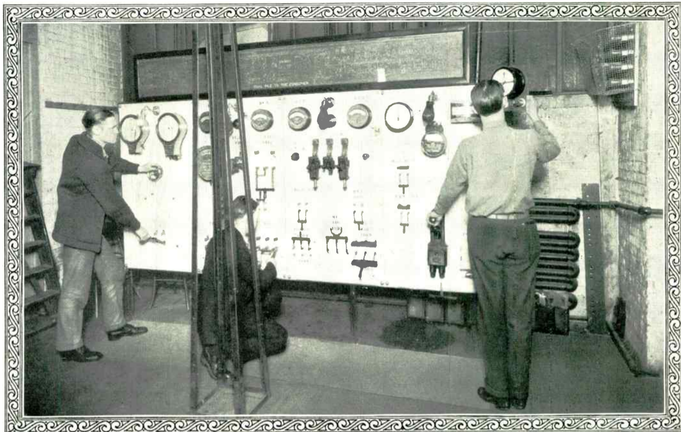
Practical Work on A. C. Switchboards. This switchboard is not "dead" but alive with "juice" and controls electrical machinery on the floor. Note the steel tower in foreground which is one terminal of high tension transmission lines, but not shown in picture.
