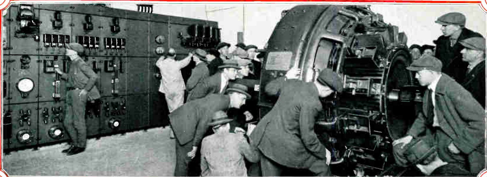
This is an automatic substation of the street railway systems, and the students are shown examining the 2000 K. W. converter, and switchboard. Trips to such plants as these are intensely interesting and inspire the student to work harder.
