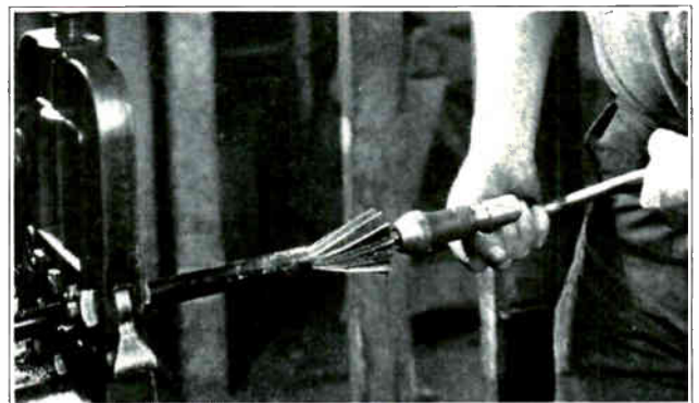
Fig. 61. Reaming the end of a piece of conduit after cutting to remove sharp edges, which might damage the insulation on the wire.
