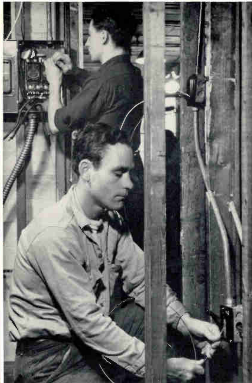
Another important part of house wiring is pulling the wires through the conduit after it has been installed. Here you see students getting practical experience on wire pulling.
