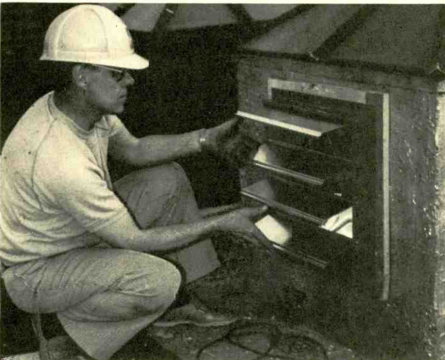
Check the operation of the self-opening louvers. Be sure that they do not bind, scrape or stick. Remove any bits of material that might cause sticking, after all you want to make certain they open everytime. Who wants to go on the roof more than they have to?
