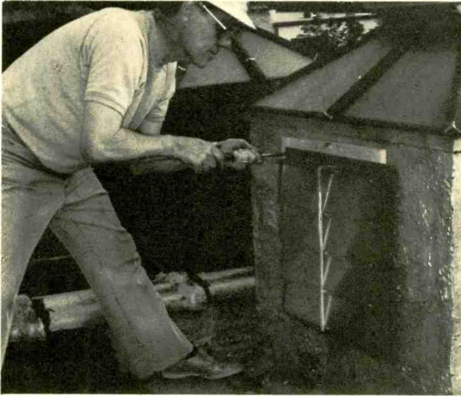
A pre-cut frame made of 3/4-inch thick wood is slipped behind the fan and secured to the wall with 2-inch long, No. 8 wood screws. The frame strengthens the wall. Now is a good time to remember a previous hint—remove all that trash off the roofing!
