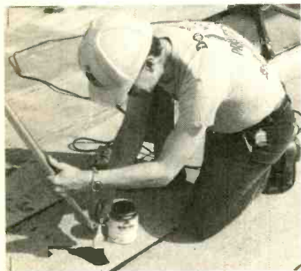
Use roof patch compound to prevent rain-water leakage through the pilot holes.
