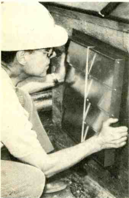
The fan fits! However, thermostats must be secured to the inside of the air duct and a wood frame made to support the fan.
