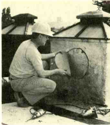
The cardboard template is pulled free and we see the drilled holes. A hammer and chisel finally freed the outlined disc.
