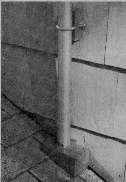
Bottom of antenna mast fits into hole drilled part way through a wedge-shaped block protecting roof shingles. U-bolts pass through wall of house into attic. Note spacer block between the mast and wall to keep the mast vertical.
