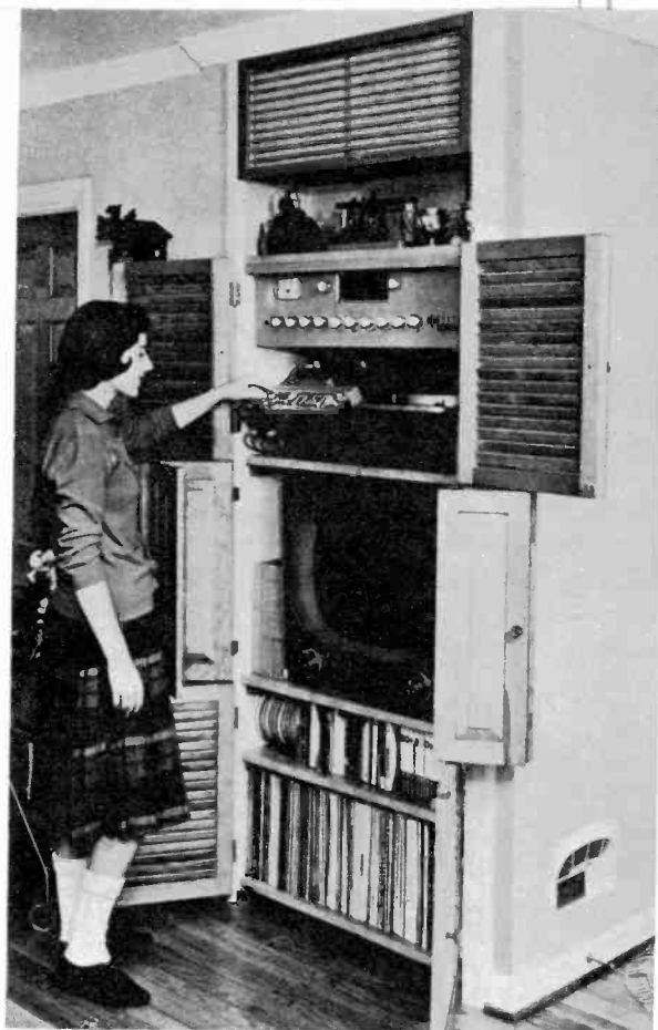
Three feet of wall space contain AR-2 enclosure, Bell 3030 stereo amplifier, Bell 2520 AM-FM tuner, Bell stereo tape deck, Garrard 301 turntable, custom auxiliary switches and VU meter.
