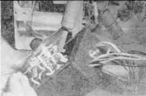
and installed in adapter box (right) between shielded lead d and switch contact 10.
