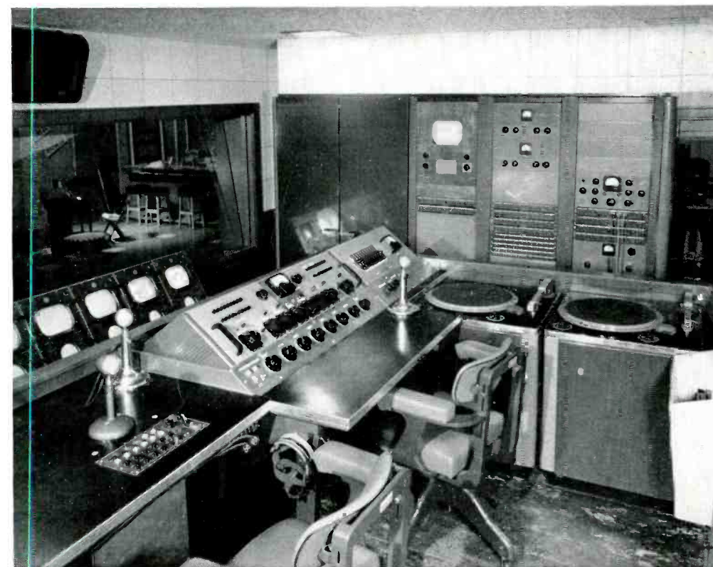
FIG. 22. View of a television studio control room showing video and audio monitoring facilities.
