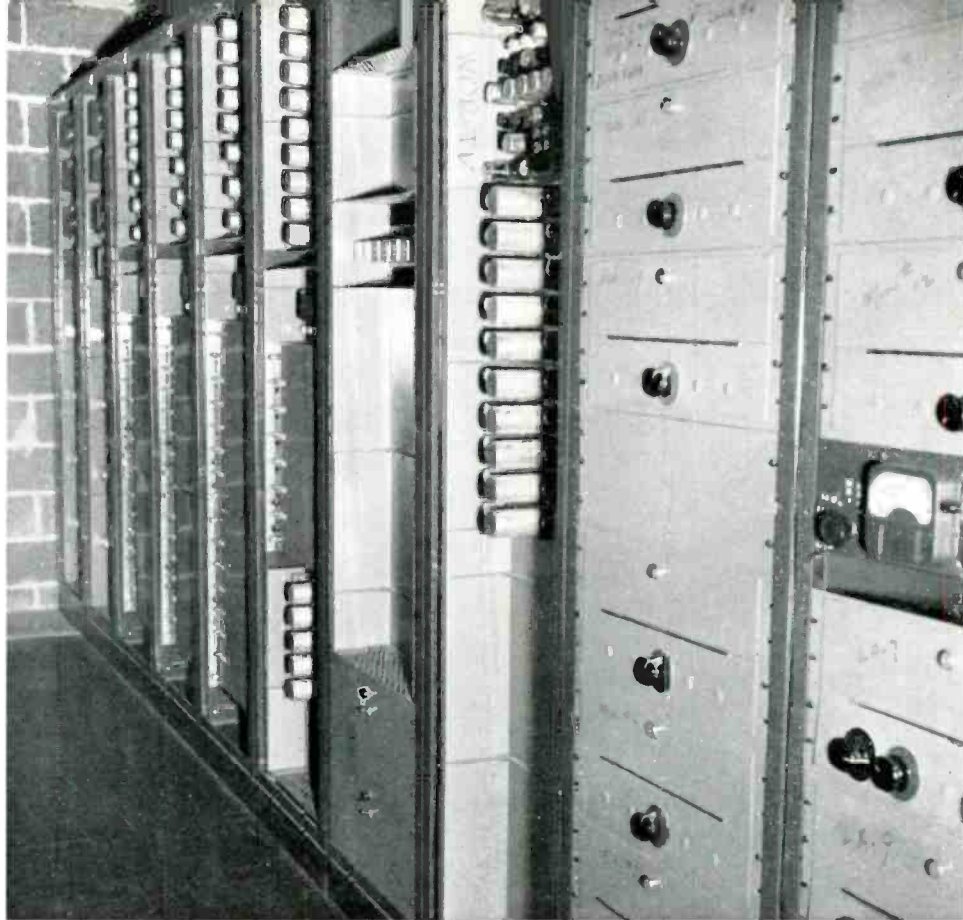
FIG. 37 (above). Second row of Master Control Racks which house TS-20A Video Switching Relays—one rack assigned to each studio system.
