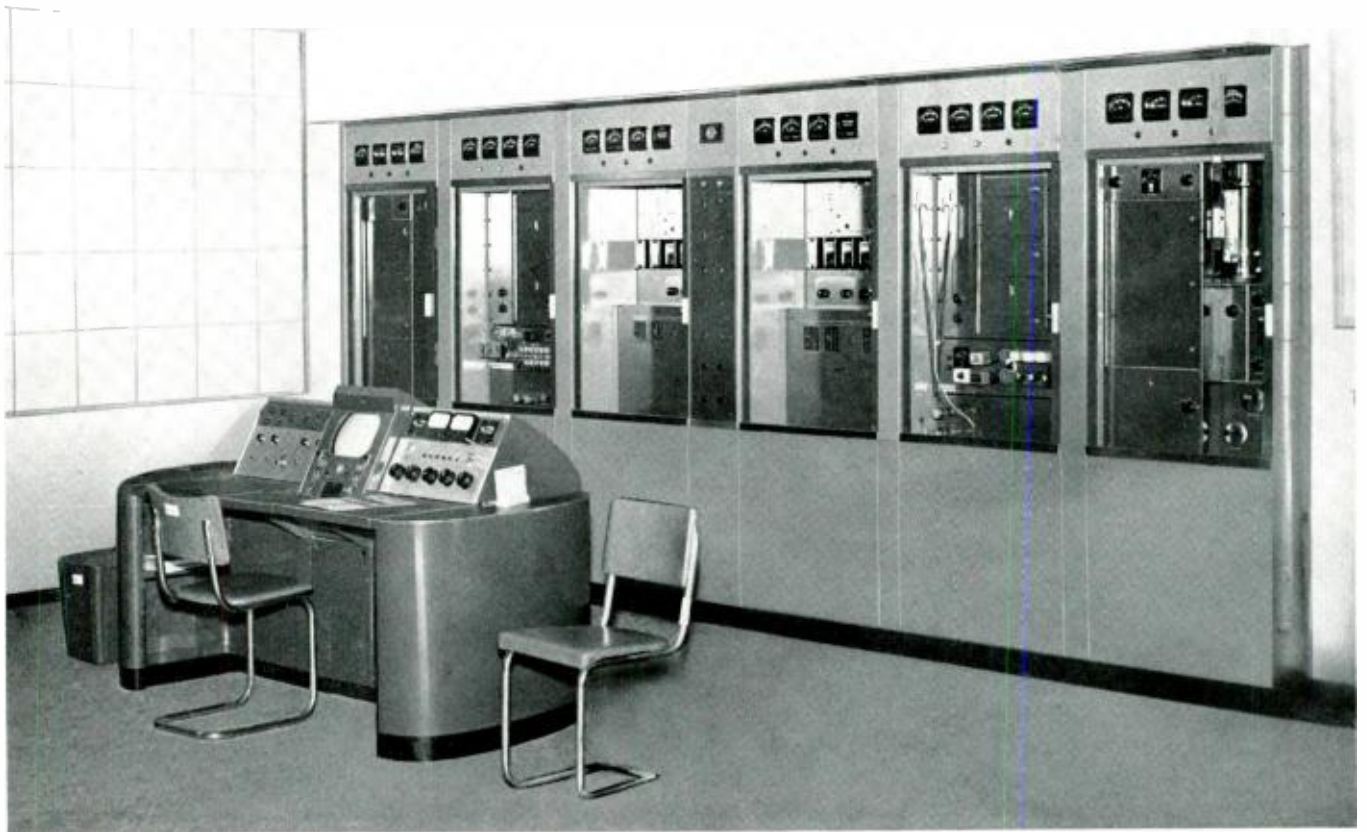
FIG. 5. Photo of typical transmitter installation showing the use of the TTC-1B Transmitter Control Console.
