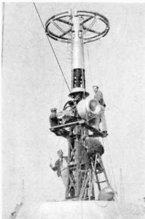
Fig. 15—Television antenna for Empire State Building during erection for test at Rocky Point Laboratory.
