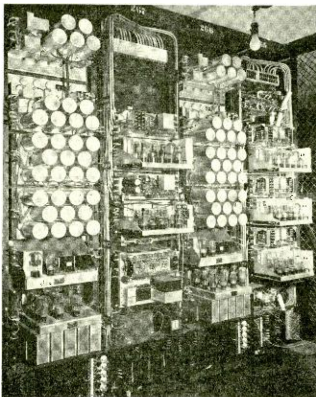
Fig. 7—Synchronizing generators and associated equipment.
