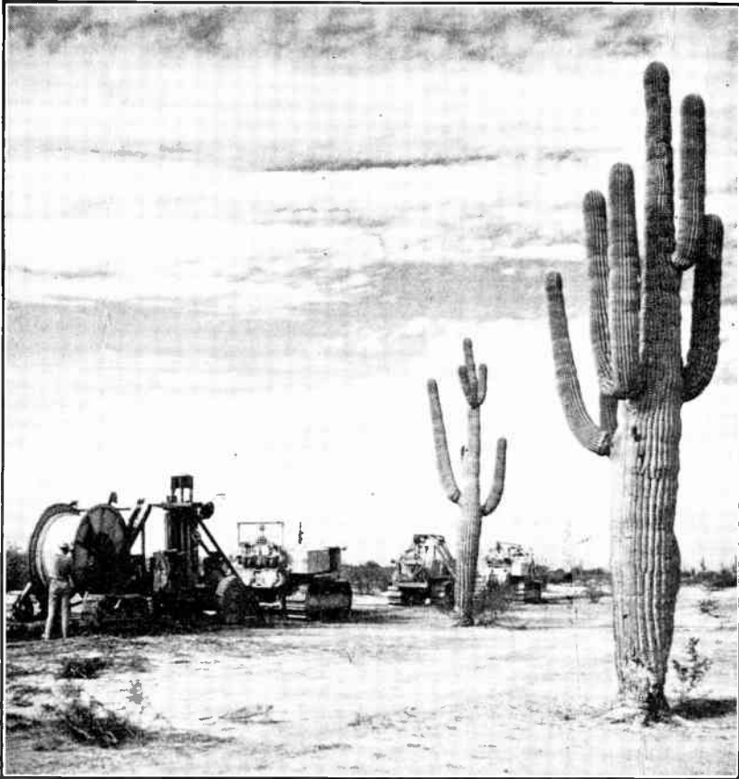
Fig. 21.28. A Cable-Laying Crew in the Desert. (Courtesy of American Telephone and Telegraph Co.)
