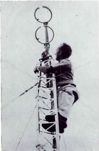
Fig. 2-15. Antenna Installation at United States Air Force TV Station, CSL-TV, Azores. The Rings are Separately Excited from Aural and Visual Transmitters. Official United States Air Force Photo.
