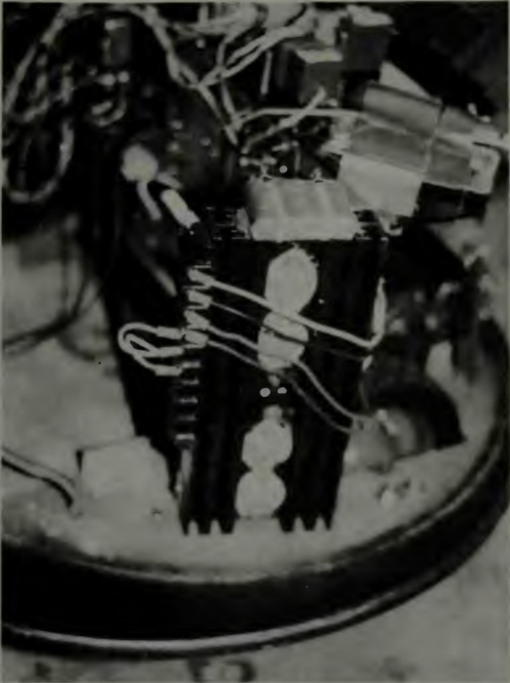
Fig. 3-14. High current motor control transistors on a heat sink base which also serves as a support structure.
