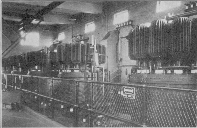
FIG. 178.—Interior view of Congress Street rectifier substation.
