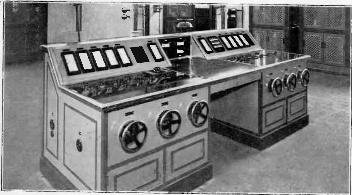
THE TRANSMITTER CONTROL DESK AT THE FRANKFURT-AM-MAIN STATION
